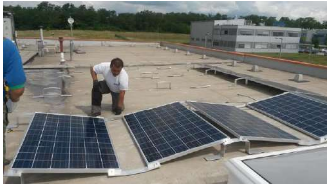
Fig. 10.b. Flat fixation of PV module installation, NVS (2014)
