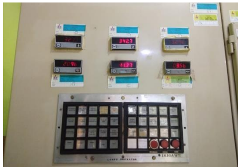
Gambar 2. Panel Kontrol Transformator
