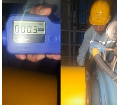
Gambar 5. Proses Pengecekan Getaran Blower
